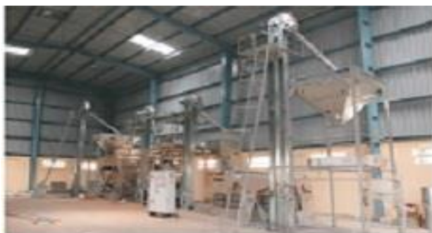
INSIDE VIEW OF PROCESSING UNIT
